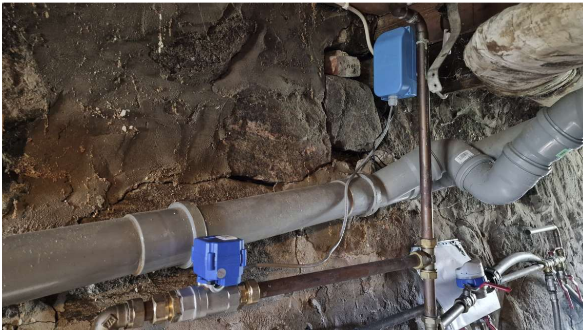
a motorized valve installed with motor facing upwards
