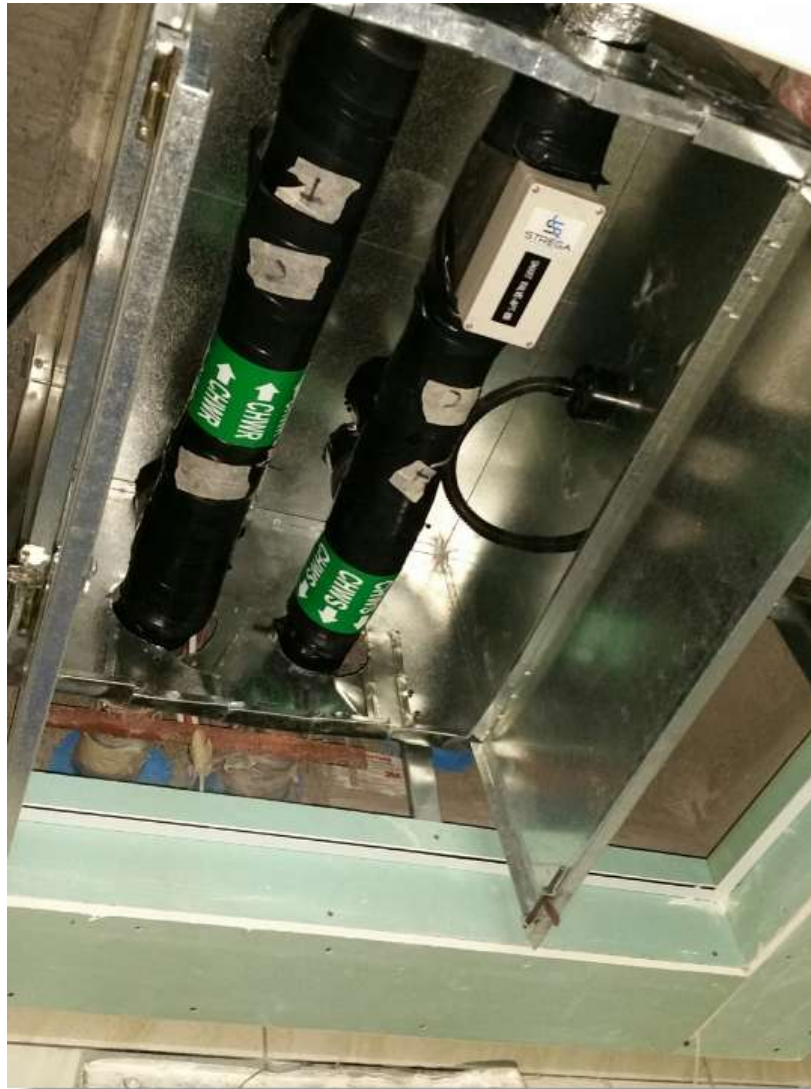
The Smart-Actuator is installed inside a cabinet in the false ceiling
